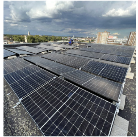
New solar panels on the roof of Hackney Empire, which were funded by the Council as part of its community energy fund
