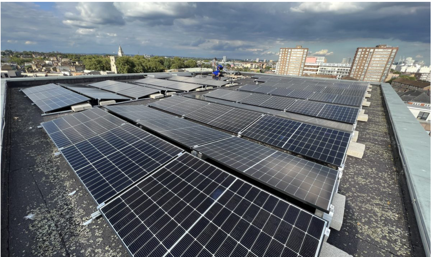
New solar panels on the roof of Hackney Empire, which were funded by the Council as part of its community energy fund
