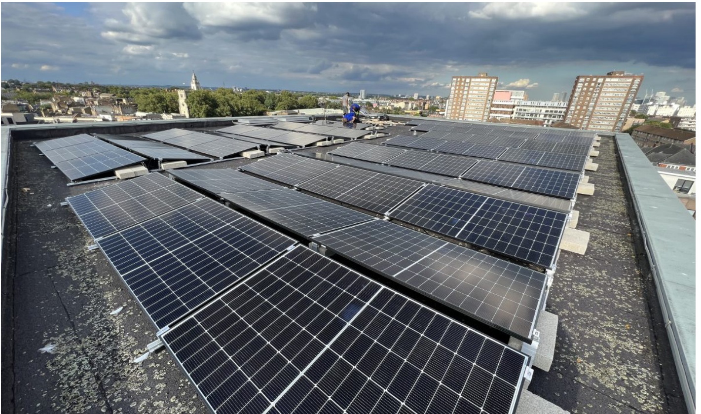
New solar panels on the roof of Hackney Empire, which were funded by the Council as part of its community energy fund
