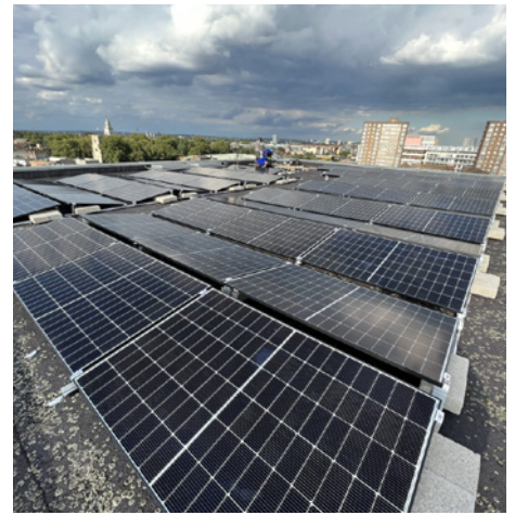
New solar panels on the roof of Hackney Empire, which were funded by the Council as part of its community energy fund
